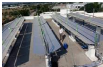
Photo courtesy: CST system installed at Zytex, Vadodra Zytex
